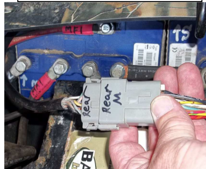
REAR Controller MASTER Under PASSENGER side
